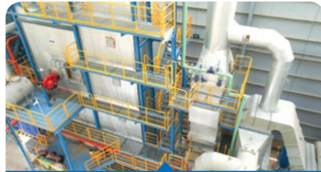
Bubbling Fluidized Bed Boiler (BFB)
