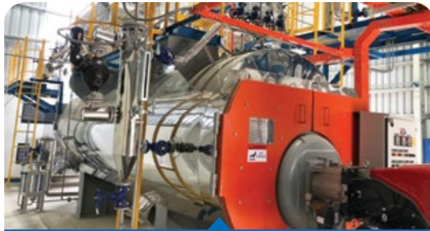
Liquid Fuel Boiler
