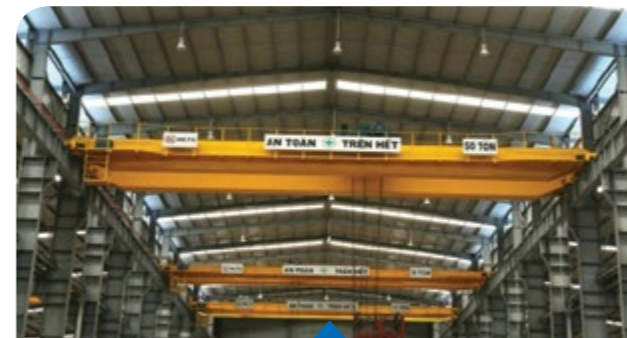
Electromagnetic Crane 50 Ton (2 units)
