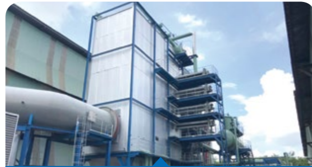
Heat Recovery Steam Generator (HRSG)
