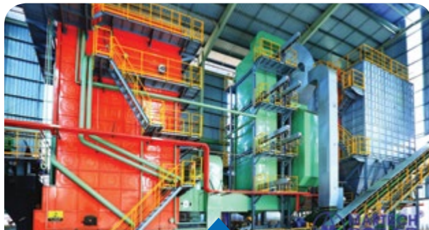
Chain Grate Boiler
