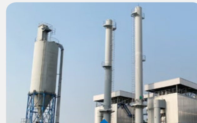
Flue Gas Treatment
