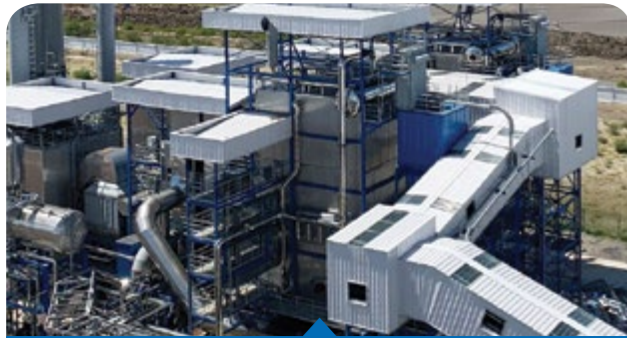
Circulating Fluidized Bed Boiler (CFB)
